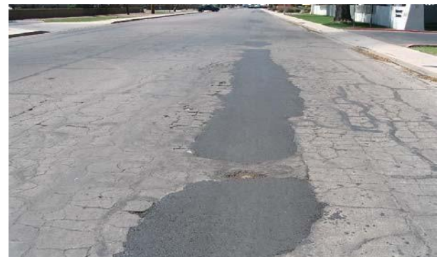
Fig. 1. (a) Pavement Condition Before the Overlay;
